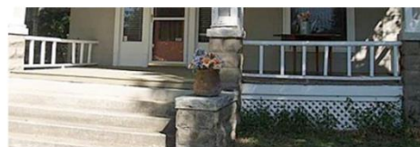
Inappropriate design! Balusters too far apart!
