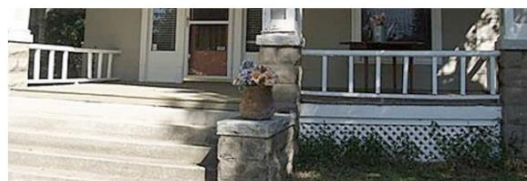
Inappropriate design! Balusters too far apart!
