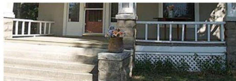
Inappropriate design! Balusters too far apart!
