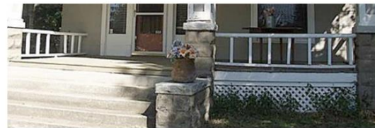
Inappropriate design! Balusters too far apart!
