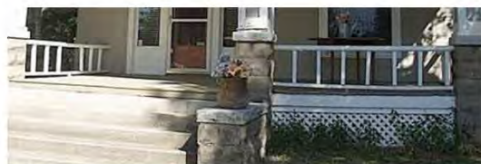
Inappropriate design! Balusters too far apart!
