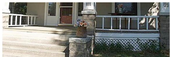
Inappropriate design! Balusters too far apart!
