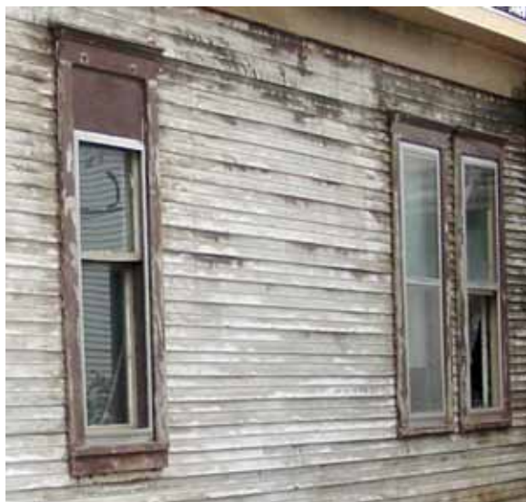
A.4.5 Inappropriate resizing, left window opening
