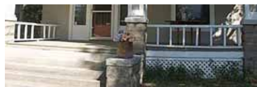
Inappropriate design – balusters too far apart.
